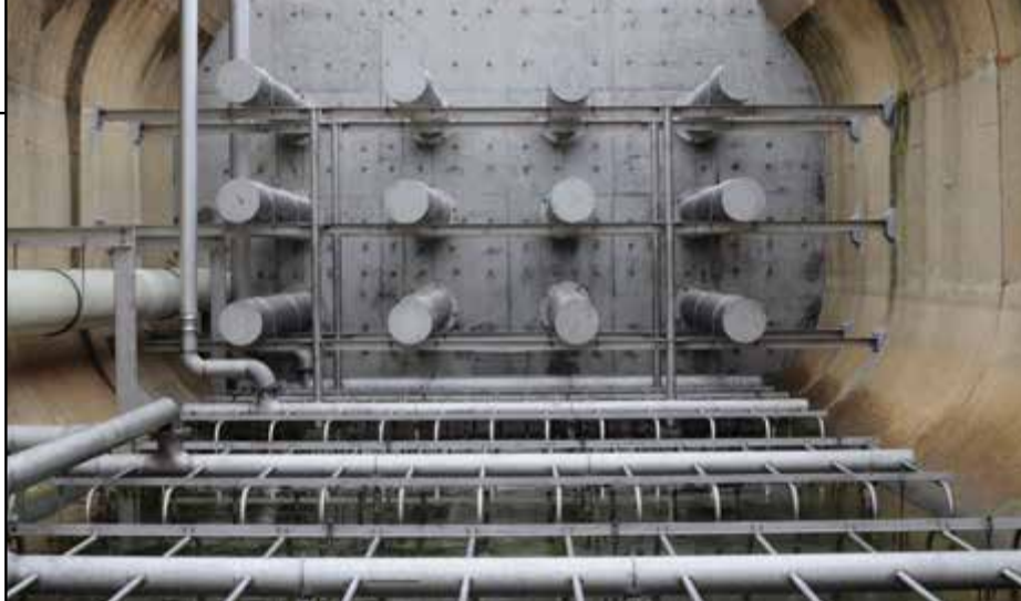
FIGURE 2. Aeration grids in the bottom of an MBBR reactor supply the oxygen needed for biomass growth
